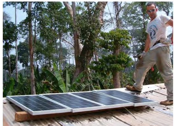
A solar home system installation like this one is cost-prohibitive for our targeted families.
